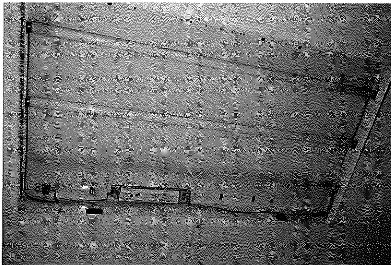
Figure 1: Building Light Fittings
