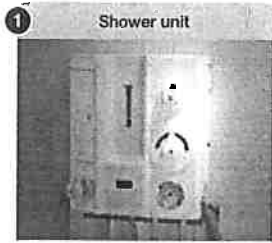
The shower unit has a thermo-static mixer and temperature display.
