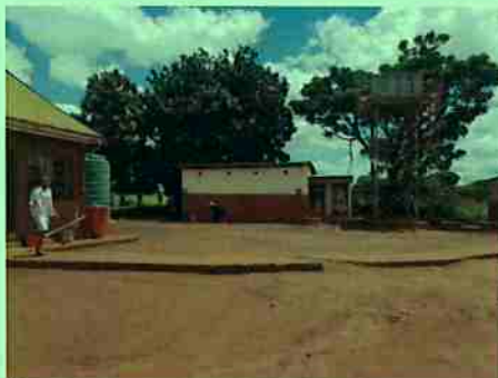
Photo 3 View of eroded external surfaces
