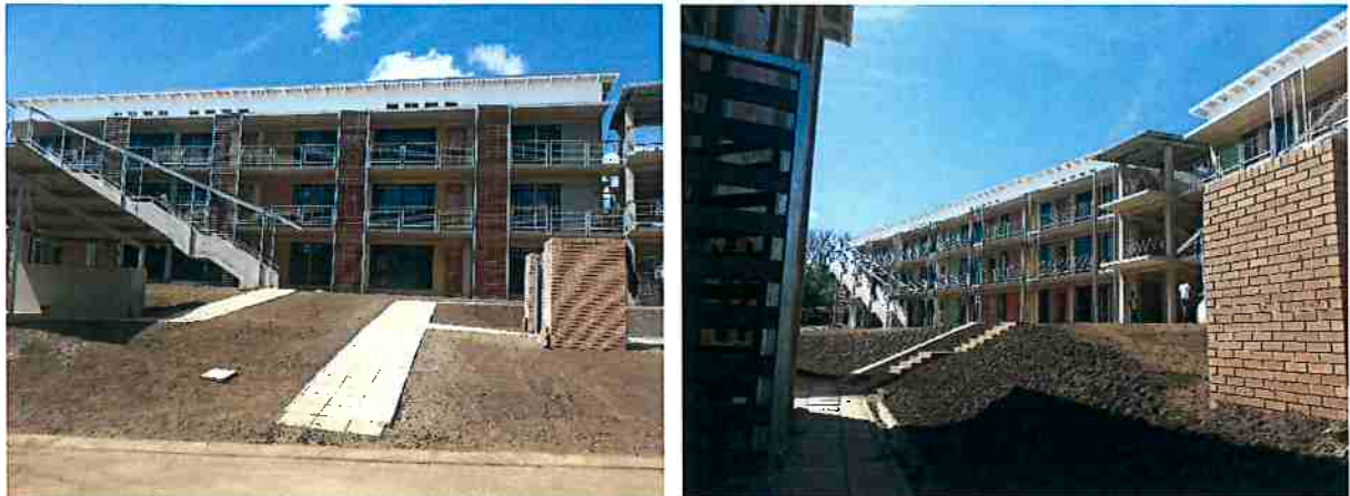
Photo 5 & 6: External views of Rietvlei Hospital Staff Accommodation (pre-occupation) SOURCE: Michelle de Goede
