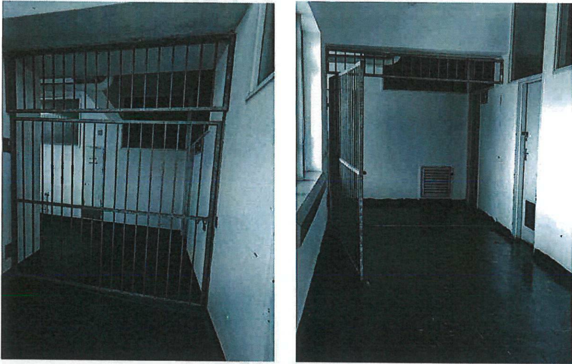
Pictures 9 & 10: Shows more burglar bars that are permanently locked, while others serve no particular purpose. The idea is to have some of the burglar bars on mag-locks that are connected to the fire protection systems. When the fire alarm sounds these mag-locks will automatically open these obstruction.
