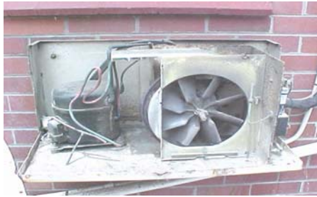
Copper wires have been removed from this air-conditioner
